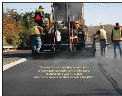
August Caption: "Paving 1/2 inch overlay on one mile of interstate on both sides (3,800 tons) in April 2003 was $136,800 whereas in August of 2008 it costs $266,000."
